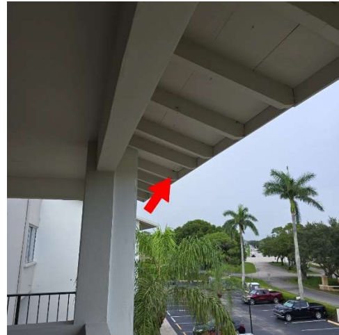
PHOTO-16 Typical Truss Fascia Rot
