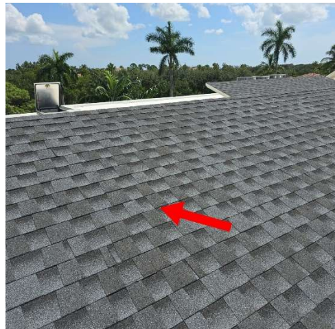
PHOTO-12 Exposed Roof Nail
