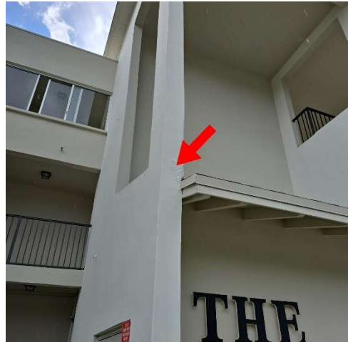
PHOTO-28 Damaged Stucco Front Entry
