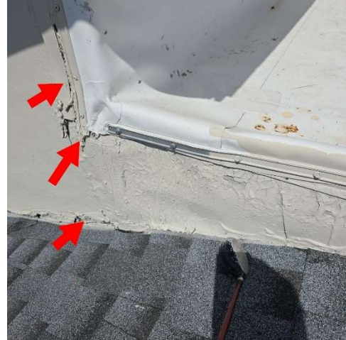
PHOTO-14 Typical Poor Roof Flashing
