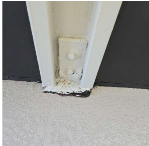
PHOTO-30 Typical Column Base Corrosion near 1B
