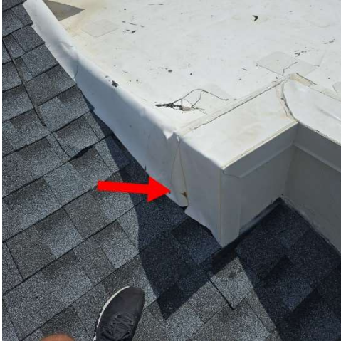
PHOTO-13 Exposed Roof Nail
