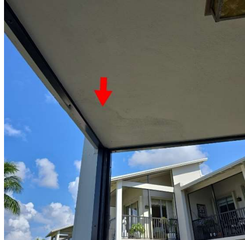
PHOTO-26 Typical Previous Concrete Repair
