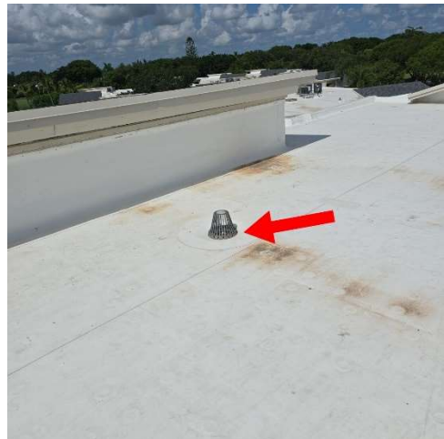
PHOTO-10 Typical Roof Drain
