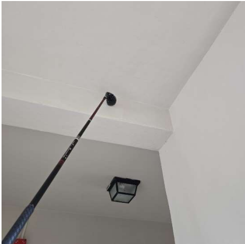
PHOTO-27 Typical Unsound Stucco
