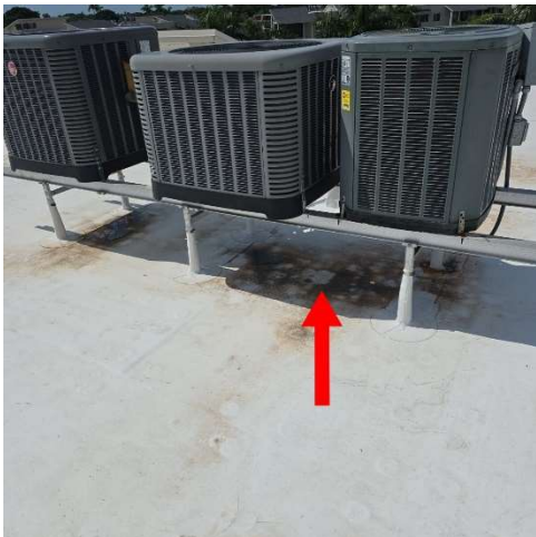
PHOTO-09 Typical Roof Staining
