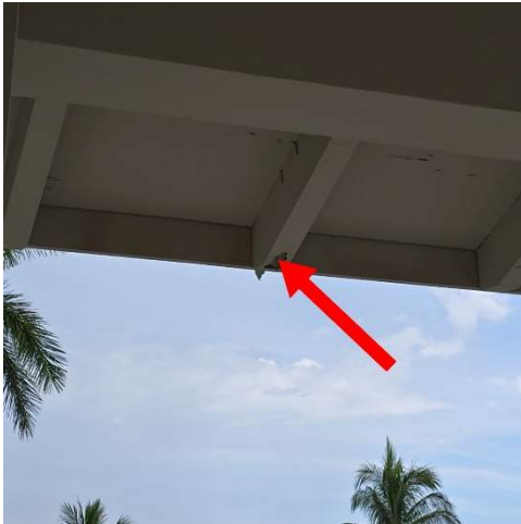
PHOTO-15 Typical Truss Fascia Rot
