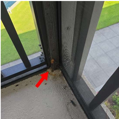
PHOTO-23 Typical Column Base Corrosion 3D
