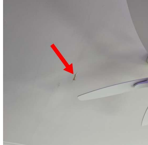
PHOTO-14 Old Ceiling Staining Unit 3F
