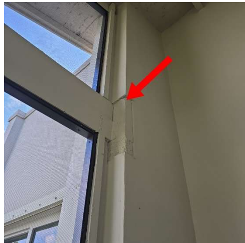
PHOTO-22 Missing Stucco Unit 3E
