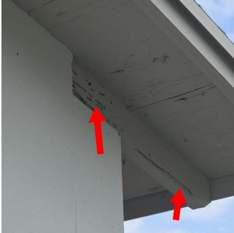
PHOTO-13 Typical Truss Fascia Rot
