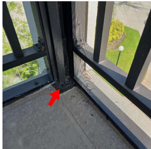
PHOTO-24 Typical Column Base Corrosion 3F
