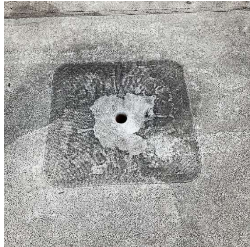
PHOTO-10 Typical Roof Drain Missing Domes
