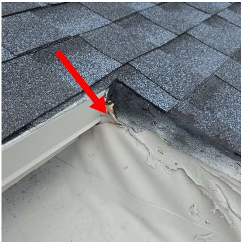
PHOTO-11 Poor Roof Flashing
