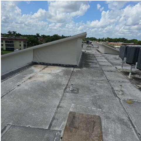
PHOTO-09 Typical Roof Staining
