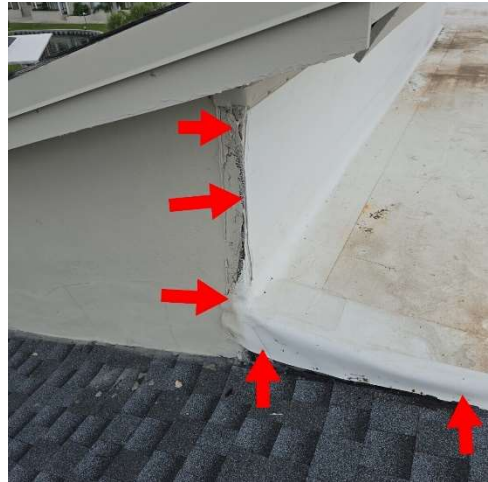
PHOTO-10 Poor Flashing and Exposed Nails
