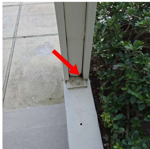
PHOTO-30 Typical Corroded Column Base near 1A
