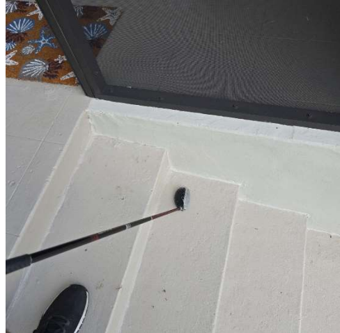
PHOTO-26 Typical Unsound Stucco near 1A
