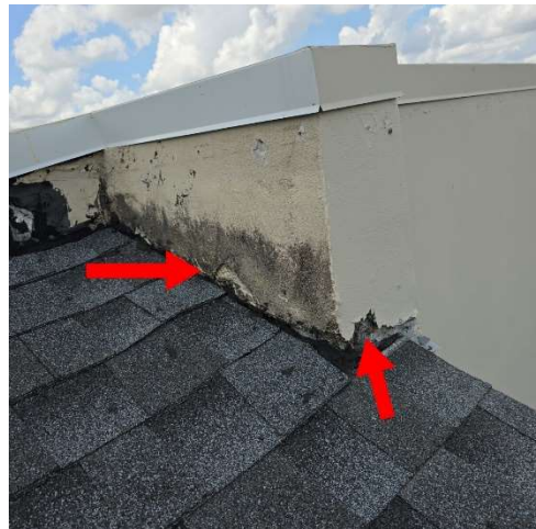
PHOTO-12 Poor Roof Flashing
