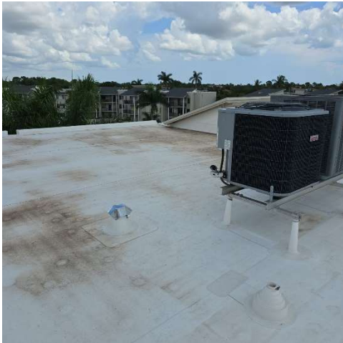
PHOTO-09 Typical Roof Staining
