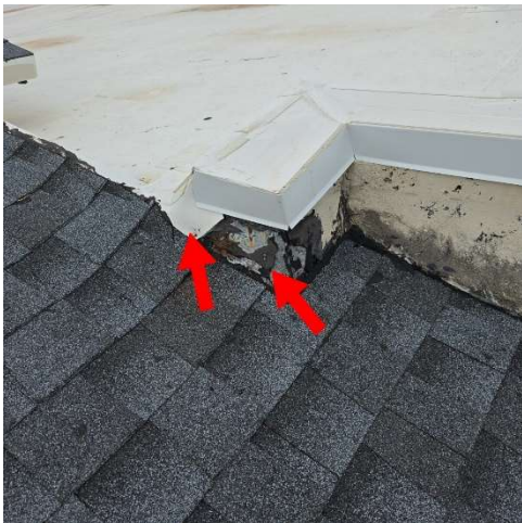
PHOTO-11 Poor Flashing and Exposed Nails
