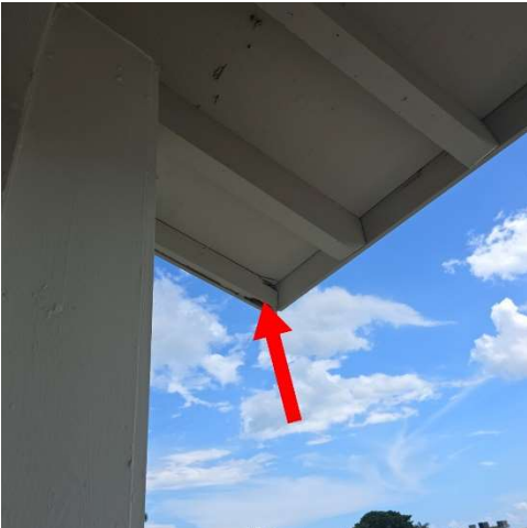
PHOTO-17 Typical Truss Fascia Rot
