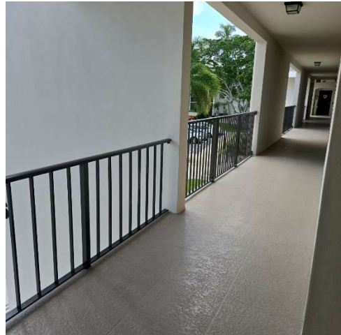
PHOTO-18 Typical Catwalk
