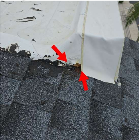
PHOTO-15 Poor Flashing and Exposed Nails
