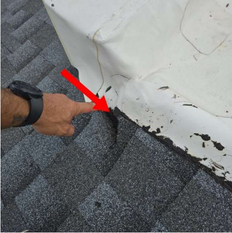
PHOTO-13 Poor Flashing and Damaged Shingle
