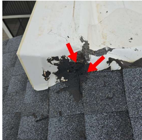
PHOTO-16 Poor Flashing Sealant
