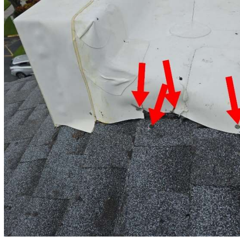
PHOTO-14 Exposed Roof Nails
