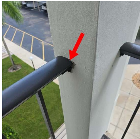
PHOTO-28 Loose Handrail to Wall Connection near 3B
