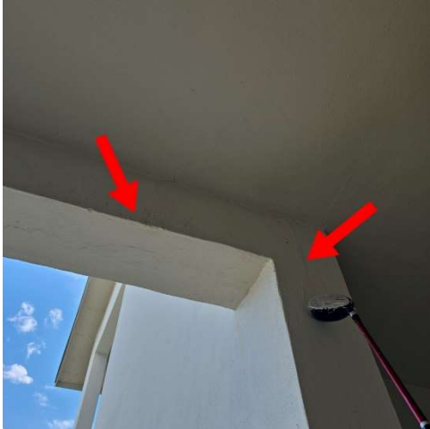
PHOTO-25 Typical Unsound Stucco and Efflorescence near 2D
