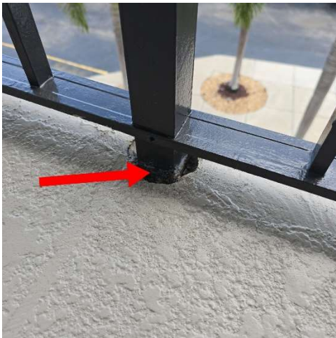
PHOTO-27 Railing Post Pocket Missing Grout near 3B
