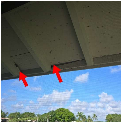
PHOTO-15 Typical Truss Fascia Rot
