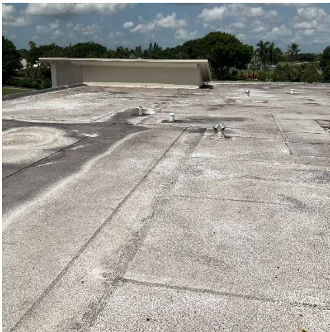
PHOTO-09 Typical Roof Staining
