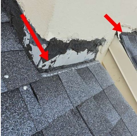
PHOTO-13 Poor Roof Flashing
