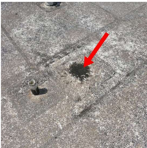
PHOTO-11 Debris at Roof Drain
