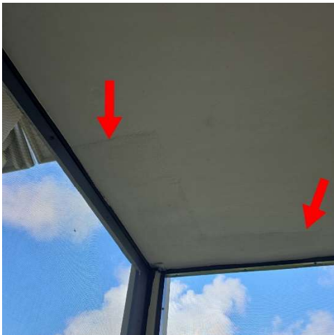
PHOTO-23 Typical Previous Concrete Repair
