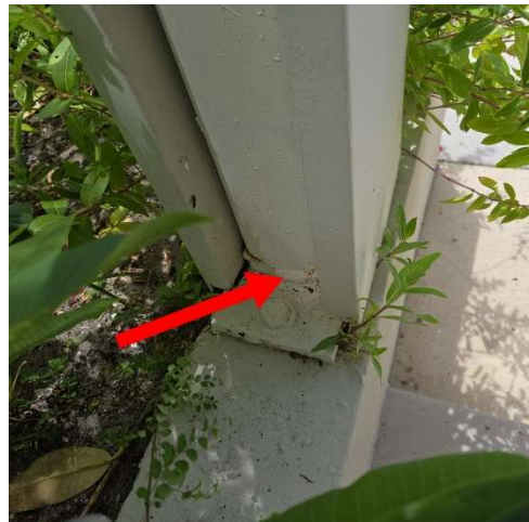
PHOTO-24 Typical Column Base Corrosion
