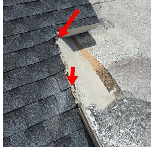
PHOTO-14 Poor Roof Flashing
