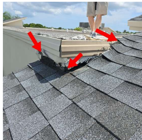
PHOTO-12 Poor Roof Flashing
